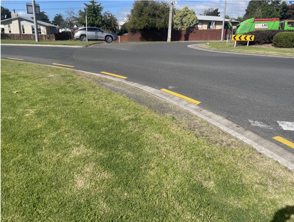
Figure 7: Skid marking indication of heavy commercial vehicle tracking encroach onto the berm area
