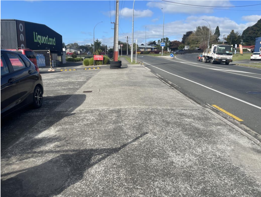
Figure 3: Large and high-use driveways on Cook Street
